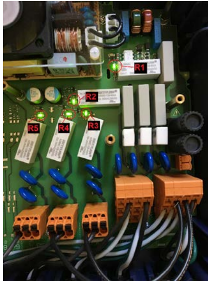
Figure 15 Internal Relays & Indicator LEDs
