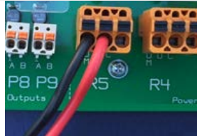
Figure 26 Remotely powered relay
