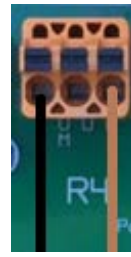
Figure 29E Concept pump cable on Output Relay R4 (Enable/Disable-ON/OFF Mode)
